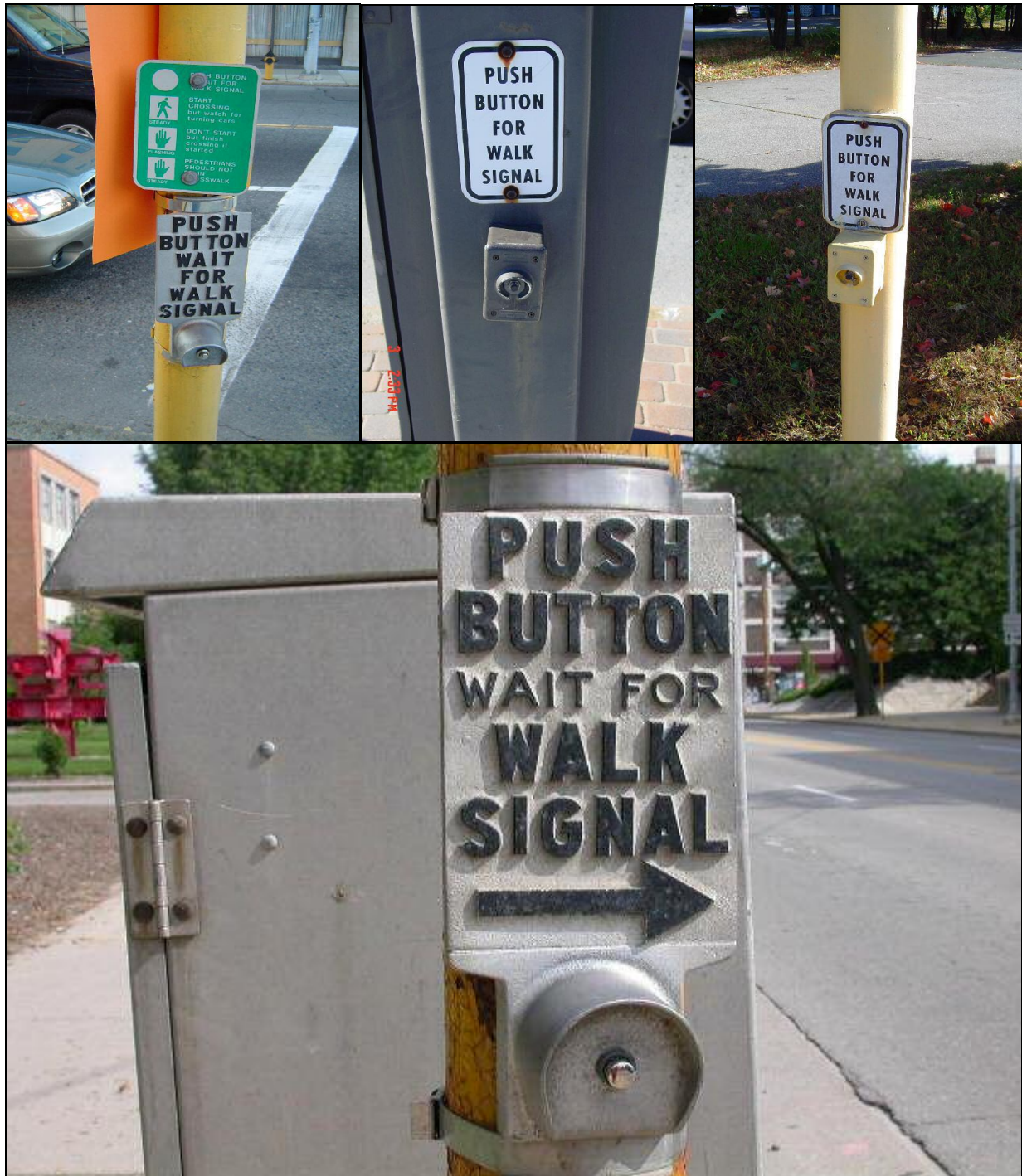
FIGURE 10 Typical Small Pedestrian Pushbuttons Used at Project Intersections.
