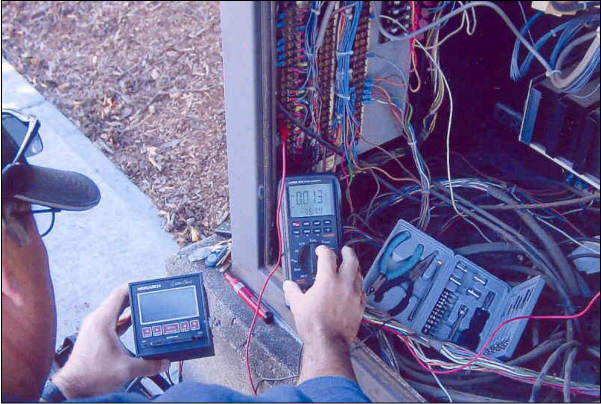
FIGURE 3 Field Testing of Cabinet Prior to Installation of Data Recorder.
